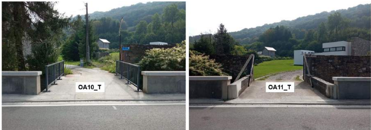
Figure 4-17 : Photo taken at the structures north of Rue Fonds de Forêt, showing the low wall on the right bank
