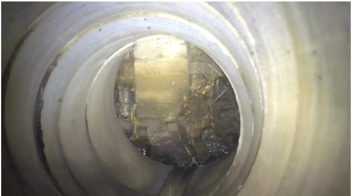
Figure 5-17 : A photo taken from the zoom showing the state of the pipe structure on Fond des Gottes.
