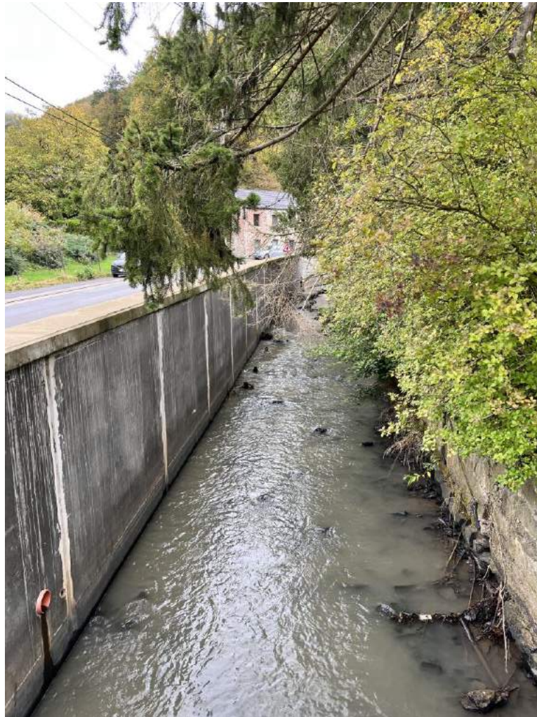
Figure 3-10 : Photo showing the low wall on the right bank of the watercourse upstream of Rue Fonds de Forêt.
