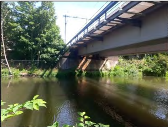
Plate 3. View looking upstream beneath the railway bridge crossing the main channel of the Roer.
