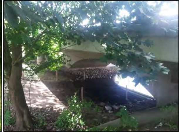
Plate 11. View of the underside of the road bridge at Site 3 from the right bank looking downstream. The river channel itself is out of view at the top left-hand-side of this photograph.
