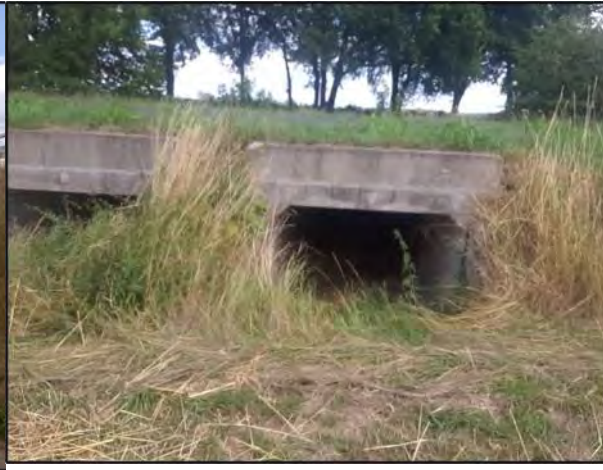
Plate 16. Exit point of the sunken box culverts which pass beneath the road north of the Roer at the Stah gauge.
