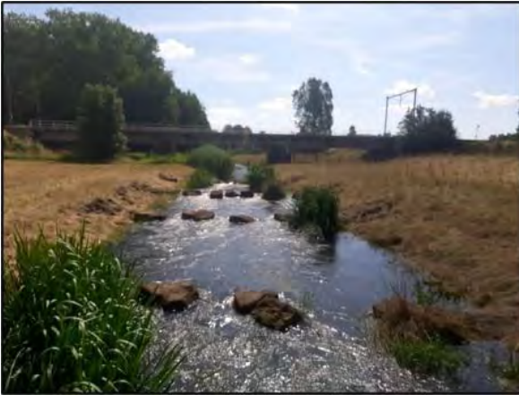
Plate 1. Looking upstream along the Groene Overlaat channel to the railway bridge. The bridge has concrete abutments and two offset piers, one on either channel bank.
